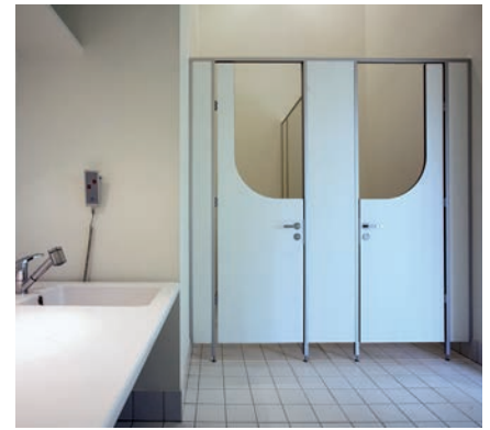
LTT 24 mm day care centre, special doors
